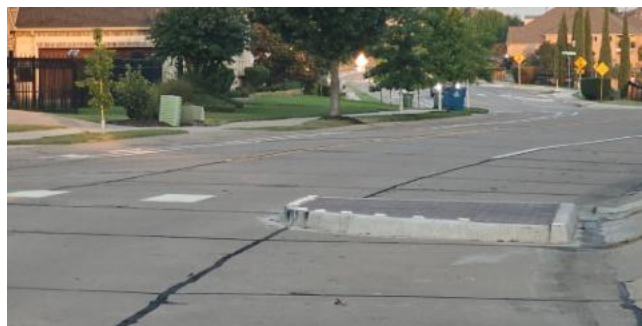
Existing bump-out has an apparent projection into the travel lane, an abrupt leading edge, and a high curb face.
