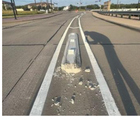
Just one example of damage to concrete separators.
